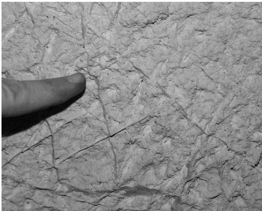
Fig. 5: Outstanding of calcite veins was formed by selective corrosion. Weathered limestone is porous and wet.
